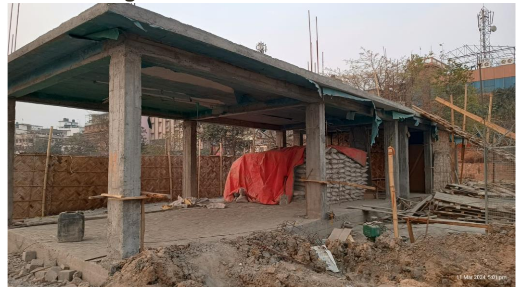
Waste Handling Station at old jail campus
